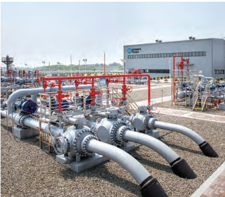
In Jintan, Changzhou, Jiangsu province, we operate an underground gas storage facility with increasing peak-shaving capability.
